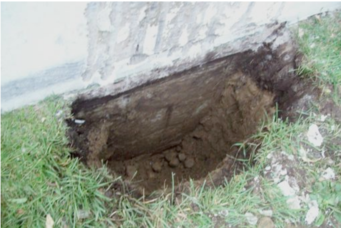
THE FOUNDATION BELOW THE WALL AT TEST CUT #1 IS OF CONCRETE BLOCK
