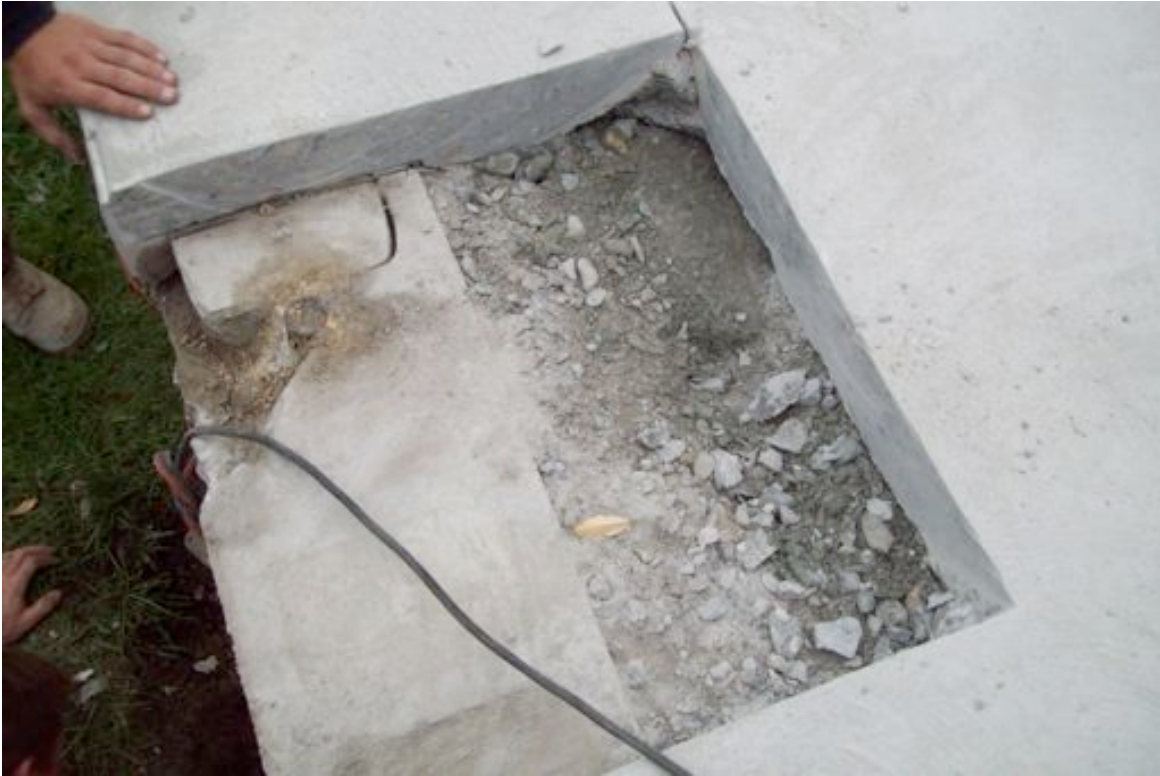
TEST CUT #1 REVEALED A BLOCK WALL
