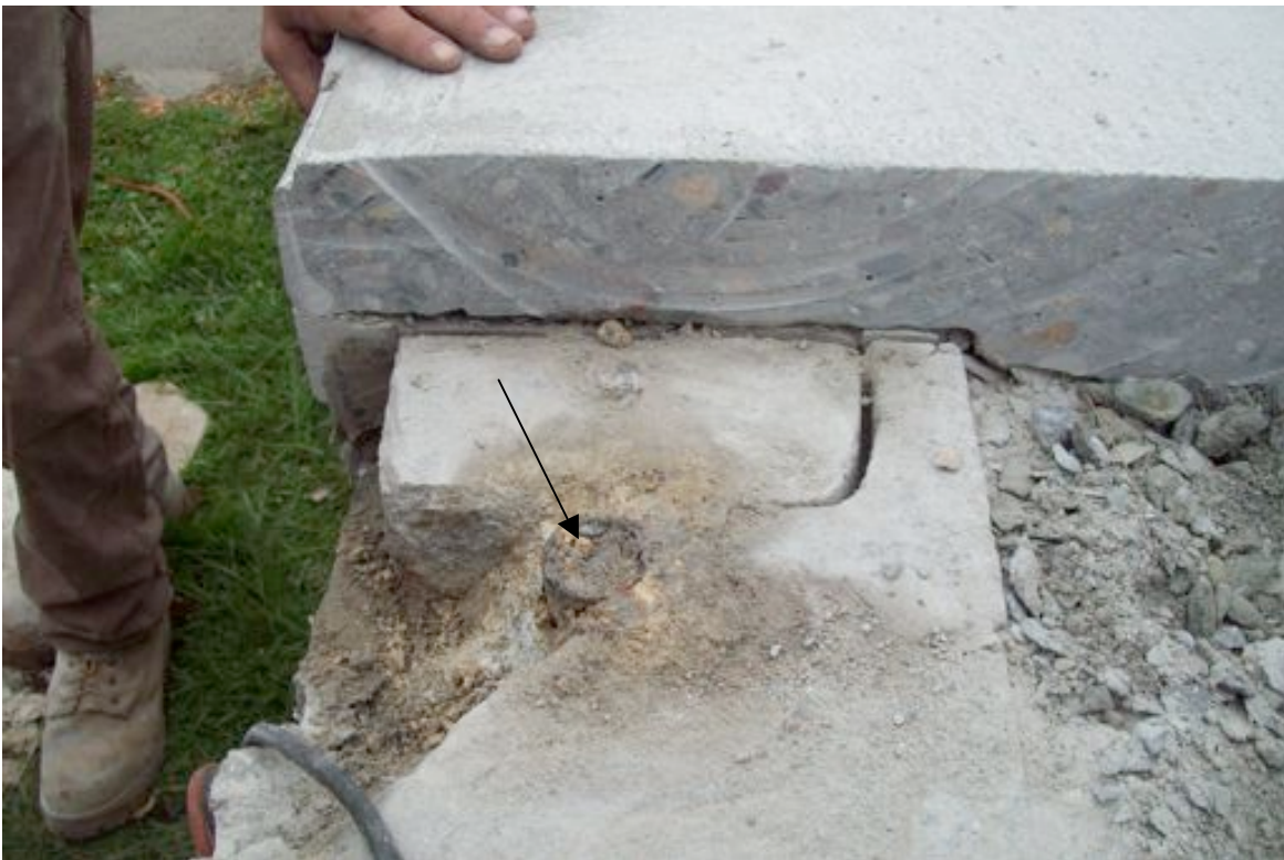
THE MAJOR DAMAGE TO THE PARGE COAT WAS CAUSED BY WATER PENETRATION THROUGH THE FENCE POST SLEEVES
