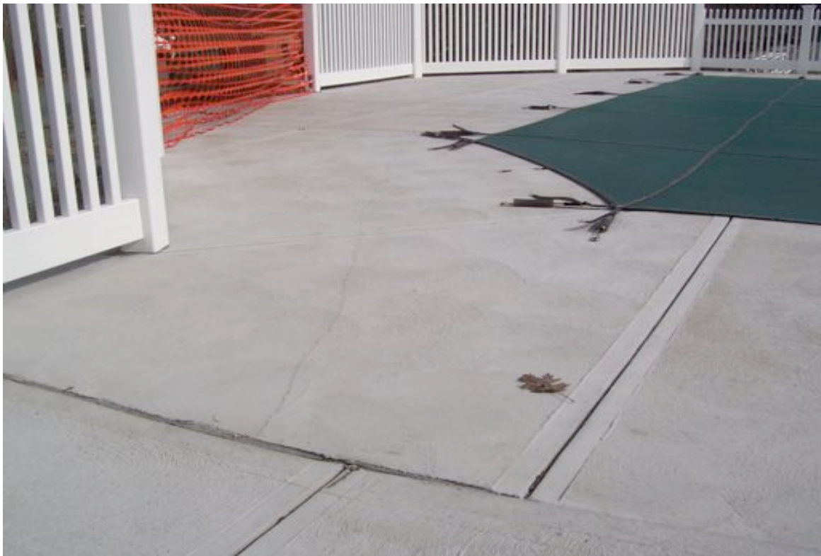
PATIO CRACKING OPPOSITE THE ACCESS RAMP EXTENDS BEYOND 4' FROM THE EDGE
