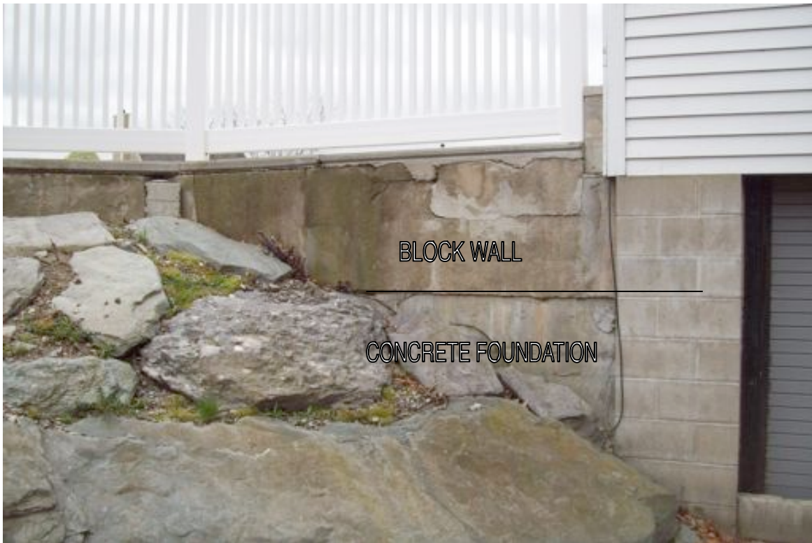
NEAR THE POOL BUILDING, THERE IS A BLOCK WALL ON A Poured CONCRETE FOUNDATION
